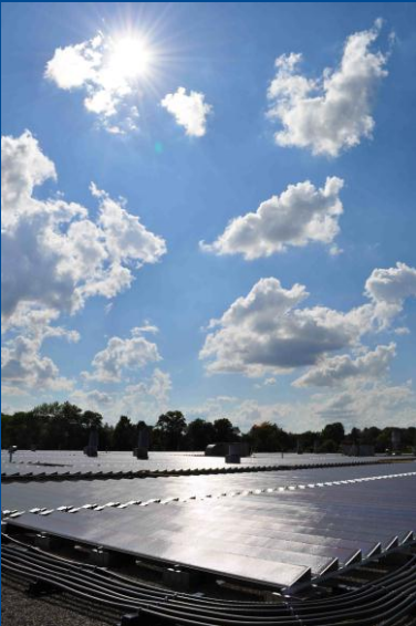
SolarShare installation in Mississauga
